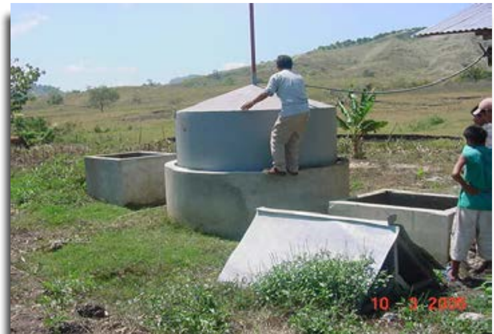
Biogas digester installed with biogas holder .
