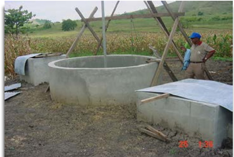
Biogas digester without the gas holder showing the inlet tank (right box) and the outlet tank (left box).
